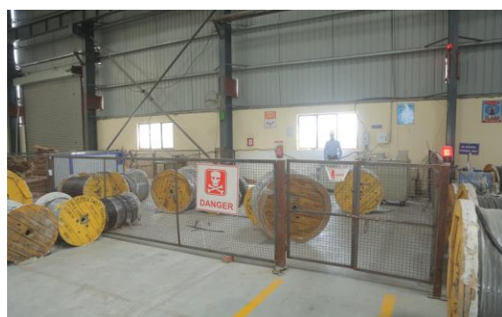
High Voltage Testing Area
